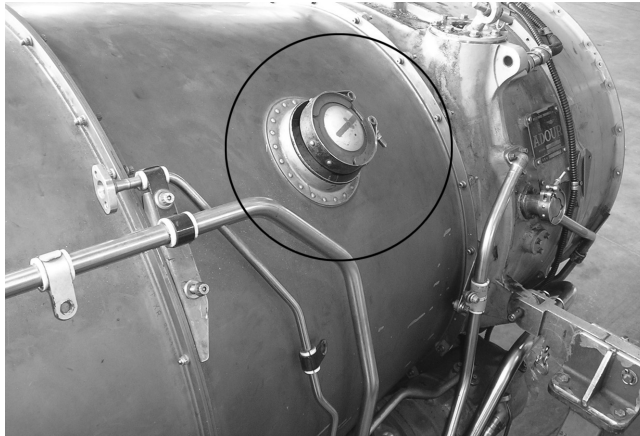
Figure 1.60 Gas turbine engine showing the outlet feed to the A/C system (courtesy of RAF Coltishall)
