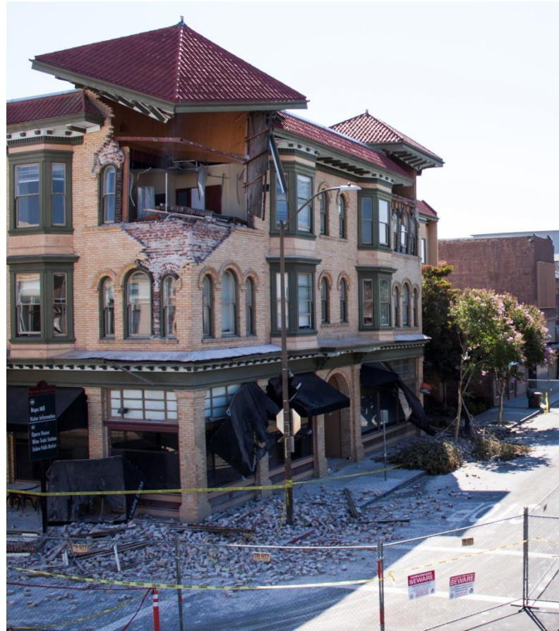
FIGURE 2.3: Napa, California, Aug. 24, 2014. This building was damaged by the magnitude 6.0 earthquake that struck Napa, resulting in a fenced-off street and closed businesses in the area. Photo by Ellis Maynard/FEMA.
