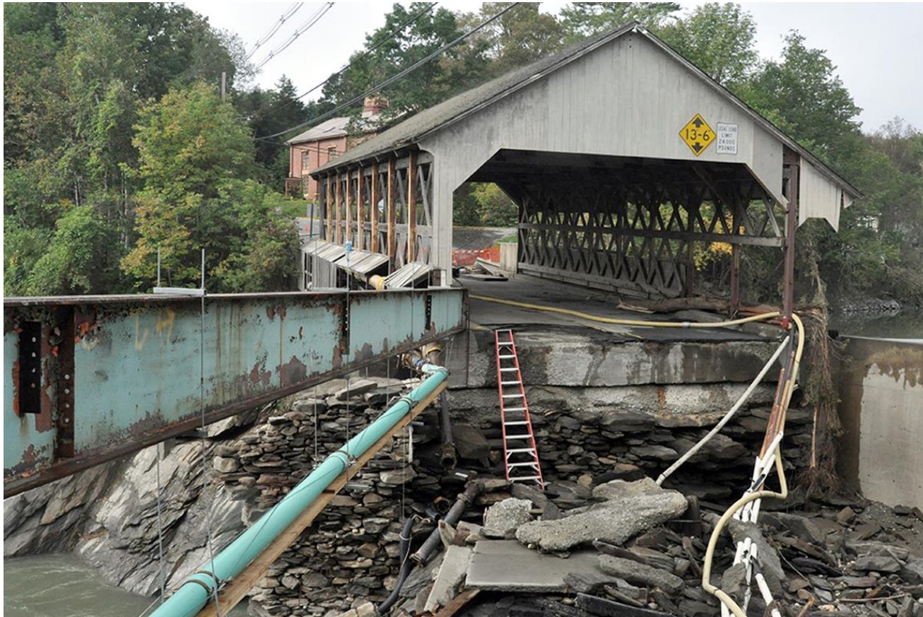
FIGURE 2.2: Quechee, Vt., Sep. 11, 2011—The Quechee bridge is a main thoroughfare and an integral part of the town. Residents cried as they watched their beloved bridge battered by flash flood waters caused by tropical storm Irene. Photo by Wendell A. Davis Jr/FEMA.
