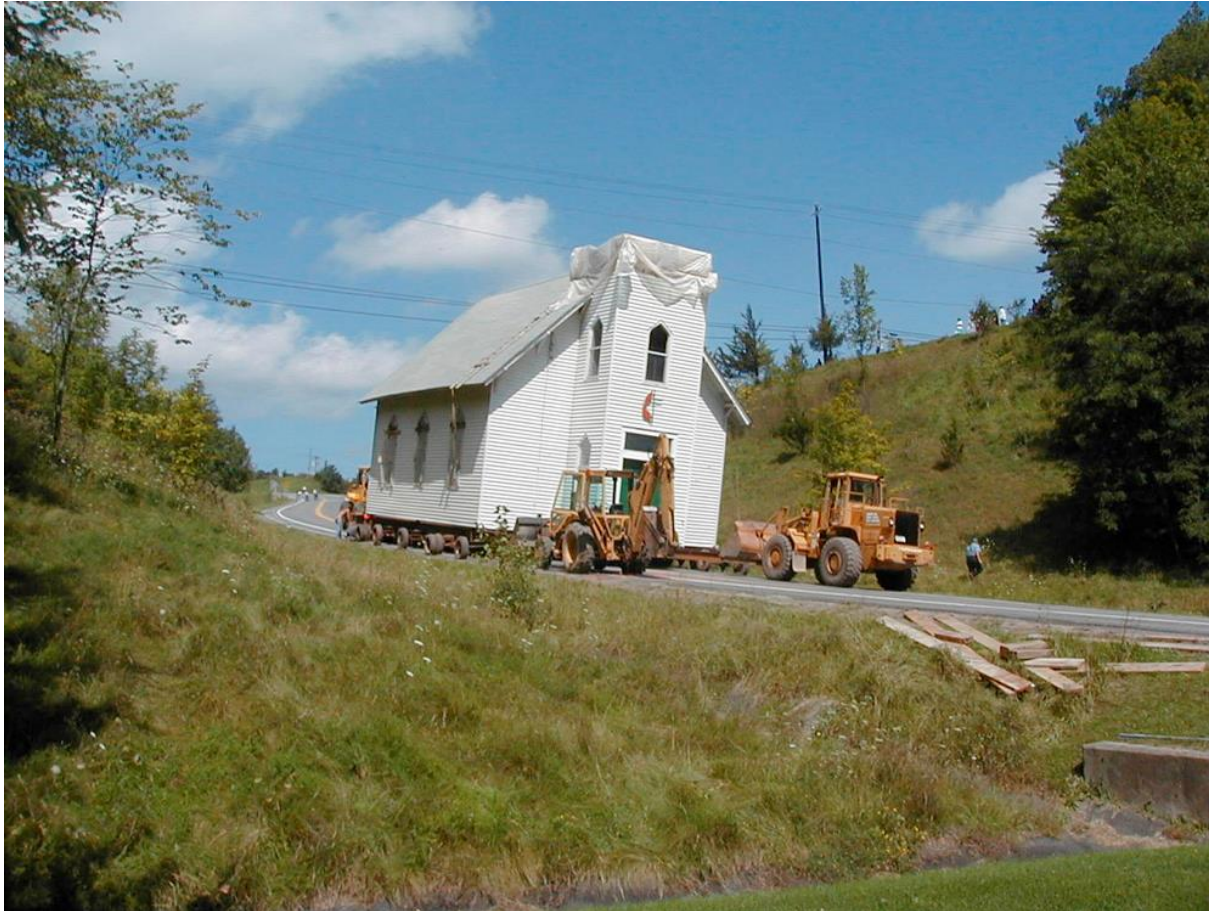
FIGURE 3.5: Albany, New York. This church is being moved half a mile to higher ground as part of the Stryker Road relocation project in Schoharie County, New York. The Hazard Mitigation Grant and Public Assistance Programs helped fund the project. Schoharie County Planning and Development Agency photos.
