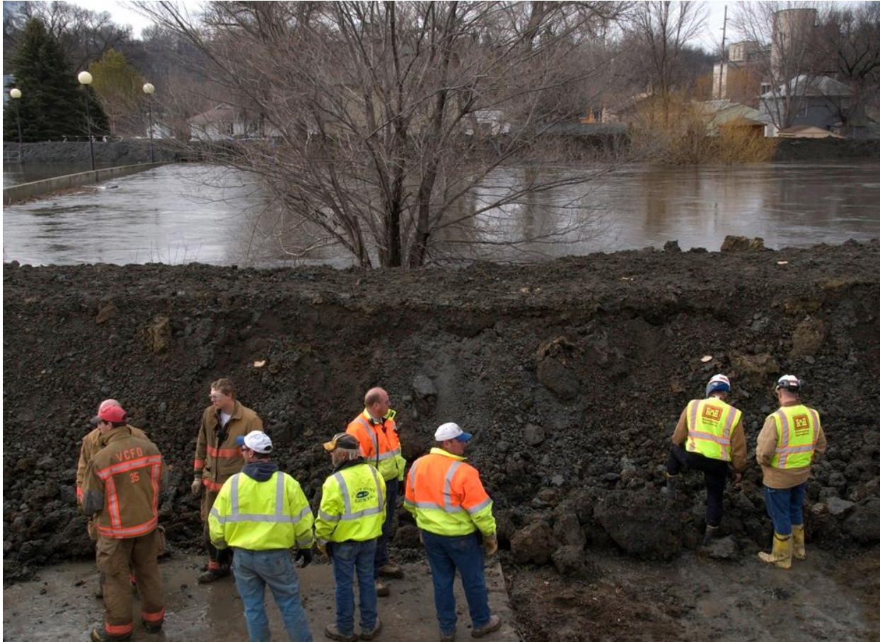
FIGURE 3.4: Valley City, North Dakota, Apr. 13, 2009. Members of the US Army Corps of Engineers inspect the site of a levee where severe seepage threatens the integrity of the levee in downtown Valley City, North Dakota. The Corps is working with city officials and the National Guard to ensure the safety of the levees in the town. Photo by Patsy Lynch/FEMA.
