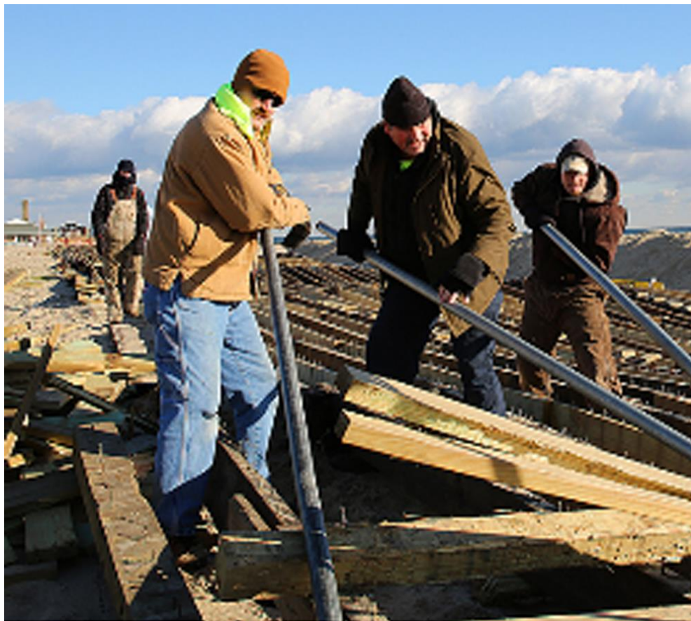
FIGURE 6.3: Asbury Park, N.J.—The Calvary Chapel Relief volunteers, a FEMA Voluntary Organizations Active in Disasters (VOAD) organization, works tirelessly on the Asbury Park boardwalk removing damaged boards while prepping the walk for the installation of new boards. VOAD is the forum where organizations share knowledge and resources throughout the disaster cycle to help disaster survivors and their communities through recovery.
