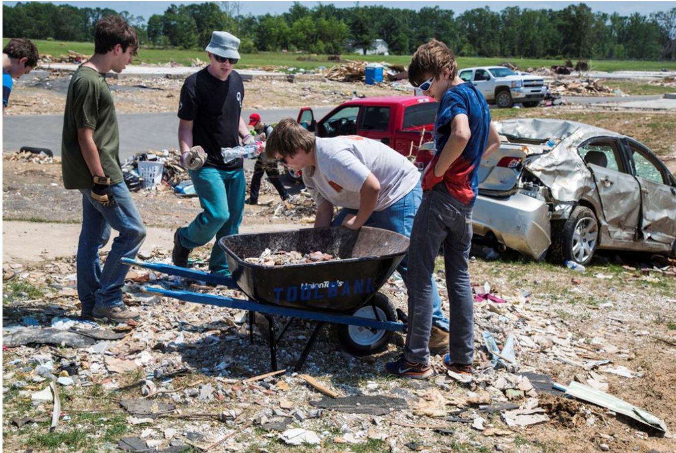
FIGURE 7.6: Vilonia, AR, May 21, 2014—Team Rubicon volunteers remove debris from a home and property in Parkwood Meadows near Naylor Road after the home was destroyed by a tornado on Apr. 27. FEMA supports Voluntary Organizations Active in Disaster (VOAD) as they help survivors recover from natural disasters. Photo by Christopher Mardorf/FEMA.
