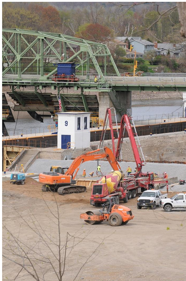
FIGURE 7.2: Glenville, New York, Apr. 18, 2012—Infrastructure on Lock-9 of the Erie Canal system on the Mohawk River is being repaired for flood control systems announced by Governor Andrew Cuomo as part of a state-wide works project. FEMA plays a vital role supporting state, tribal, and local governments as they respond with recovery efforts. Hans Pennink/FEMA.
