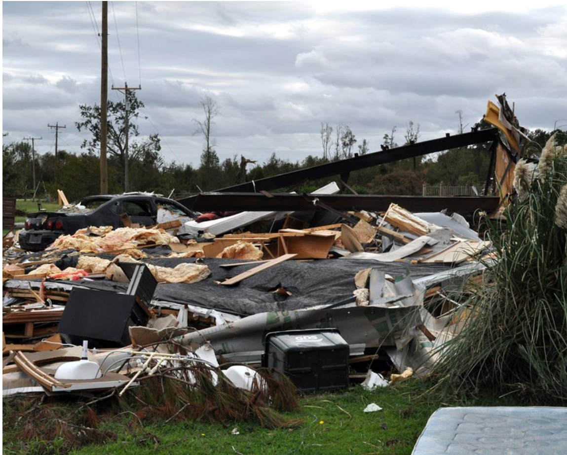
FIGURE 7.1: Columbia, N.C., Sep. 16, 2011—All that remains of this home following the EF2 tornado is the framing steel and scattered belongings. FEMA is in the area providing assistance to survivors. Marilee Caliendo/FEMA.
