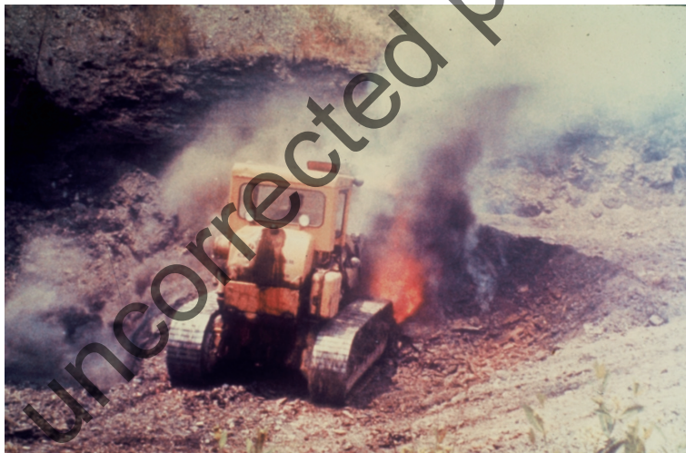
Figure 1.2.5. Excavation involves the hazards of working in hot material and toxic fumes. US Bureau of Mines photo 1982, Calamity Hollow Burnout Control Project.
