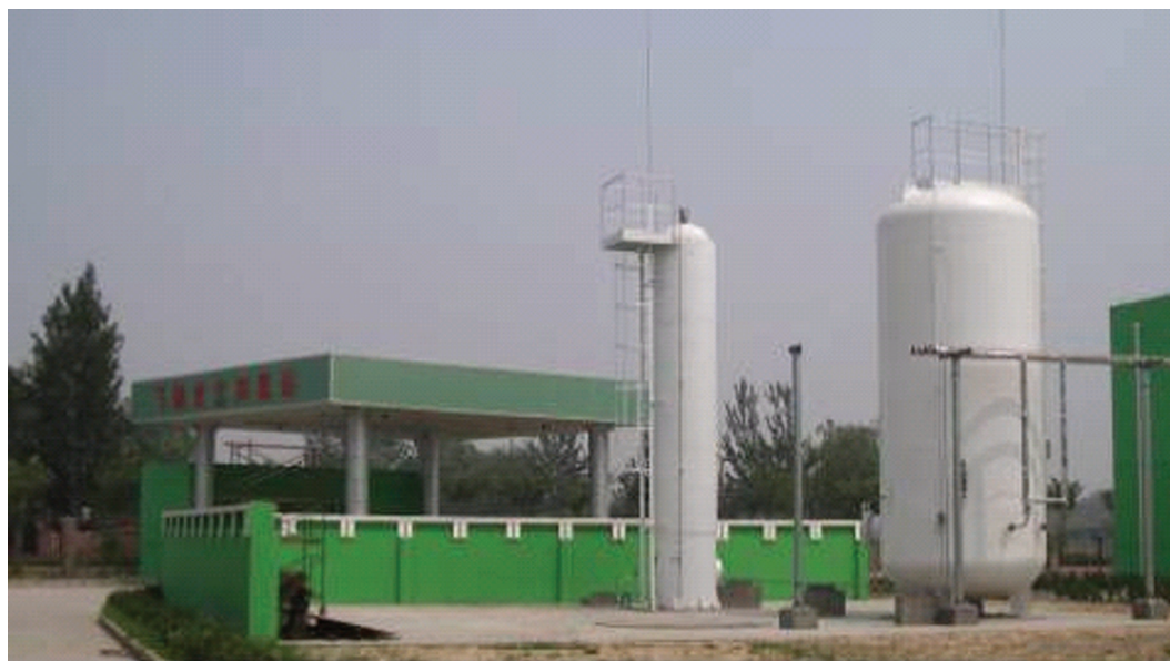
Figure 11 Picture of a hydrogen generation and refueling station. Courtesy of Beijing LN Power Sources.
