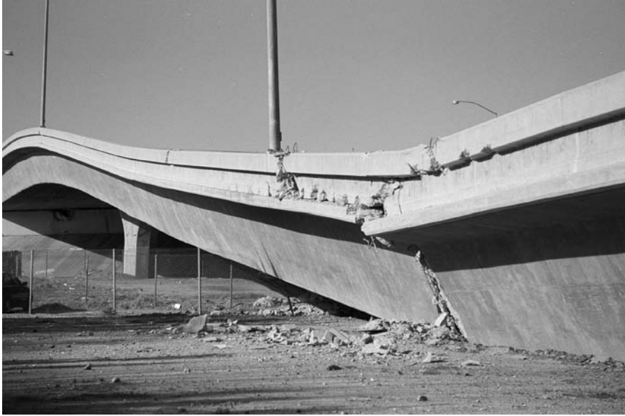
FIGURE 1–2 Northridge, California, earthquake, January 17, 1994. Many roads, including bridges and elevated highways, were damaged by the 6.7 magnitude earthquake. Approximately 114,000 residential and commercial structures were damaged and 72 deaths were attributed to the earthquake. Damage costs were estimated at $25 billion. FEMA News Photo.
